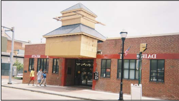
Renovations of the Cross Street Market begin at the Light Street entrance.
